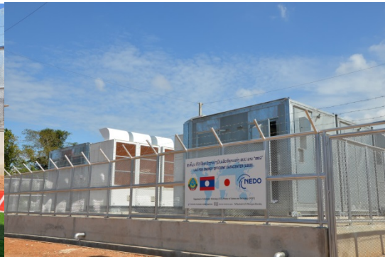
Exterior view of Lao PDR's first eco datacenter
